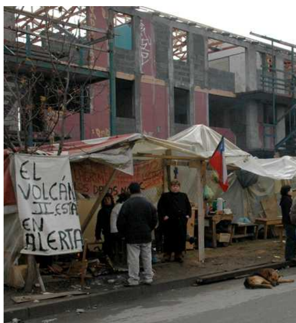
Figure 3: Ruined Houses due to faults in the fulfilment of building standards. Villa El Volcán, Santiago. Source: www.liberacion.cl
