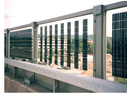
Illustration 5: Sound insulating wall with PV-modules at a motorway. [Kohlhauer GmbH]
