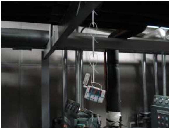
Figure 7: Thermal Recorder for the Comp. room
