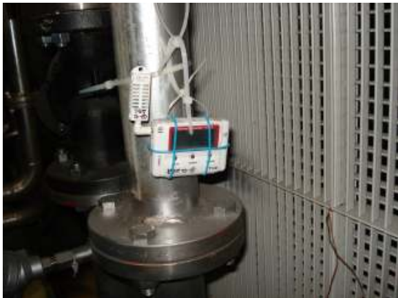
Figure 6: Thermal Recorder for the supply air of the Comp. room
