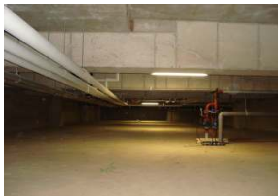
Figure 2: Cool tube of the Pit
