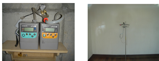
Figure 5: View of installation of measurement units
