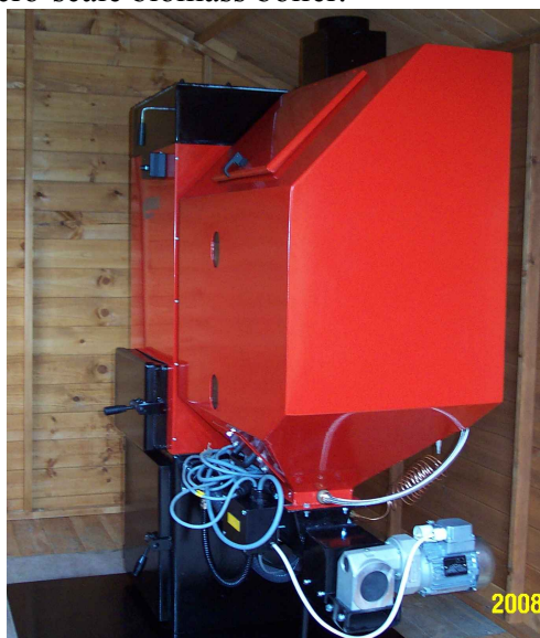
Figure 4: 25kW biomass boiler designed by Ashwell Engineering Services Ltd (UK) in the University of Nottingham
