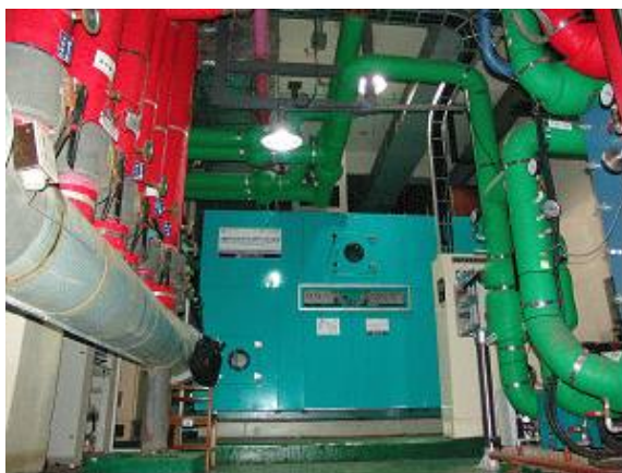
Fig. 3 Photograph of system in site
